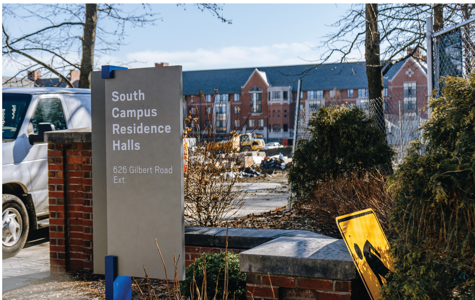
The current construction project on South Campus, which has been part of the University of Connecticut's Master Plan since 2015, involves the addition of a new residence hall. Since the building will face Gilbert Road, vehicles such as shuttles will no longer have permission to pass by that part of campus while construction is going on.
