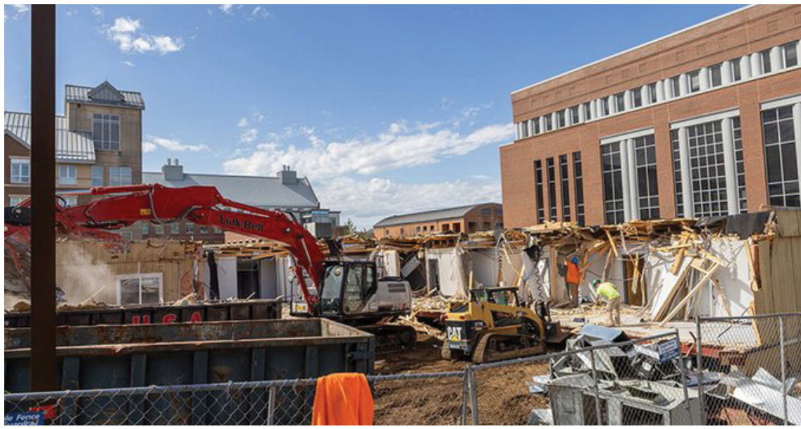
The demolition of Eastern Hall at Eastern Connecticut State University starts on April 10, 2024. After demolition, blueberry bushes and trees will be planted in Eastern Hall's place.
