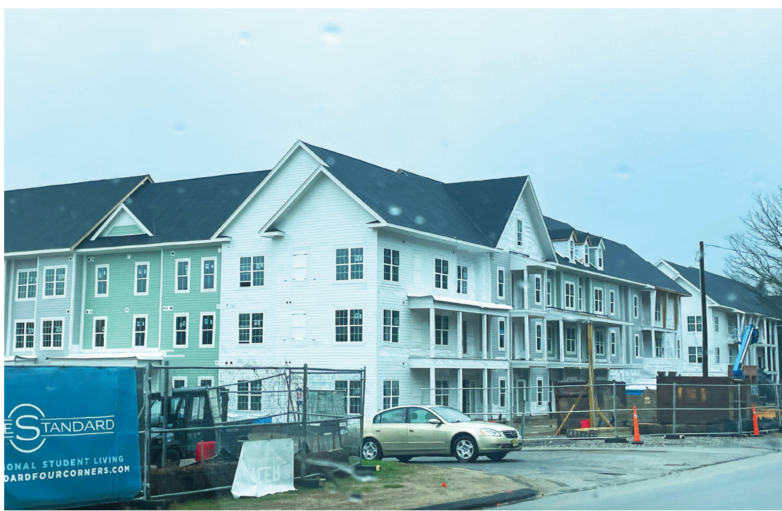
Construction continues on The Standard at Four Corners apartment complex in Storrs, Conn. on Friday, April 12, 2024. The development will offer housing to University of Connecticut students as well as the general public and are expected to open in Fall 2025. PHOTO COURTESY OF THE AUTHOR
