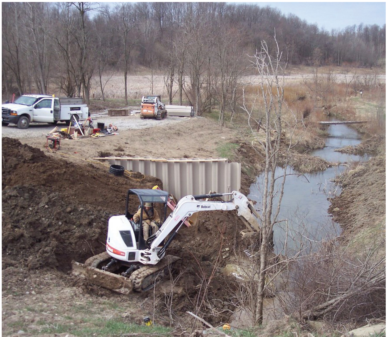
Construction of a ditch plug for wetland restoration. The proposed revisions of the term "waters of the United States" could leave 85% of wetlands without any federal protection. PHOTO COURTESY OF FLICKR
